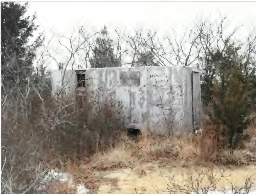
Figure 5.42. View looking north at a post World War II trailer located near Batteries Peck and Engle. The trailer is in a seriously deteriorated condition and, along with an accompanying section of fence, should be removed to improve the visual and spatial connection among Battery Peck's gun emplacements, commander station, CRF station, and the water in the distance (Olmsted Center, January 2009).
